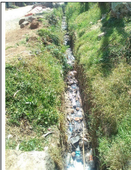
Plate 1: Blocked open ditch
